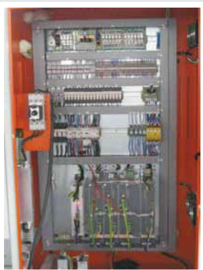
CE-Marked Electric Cabinet
